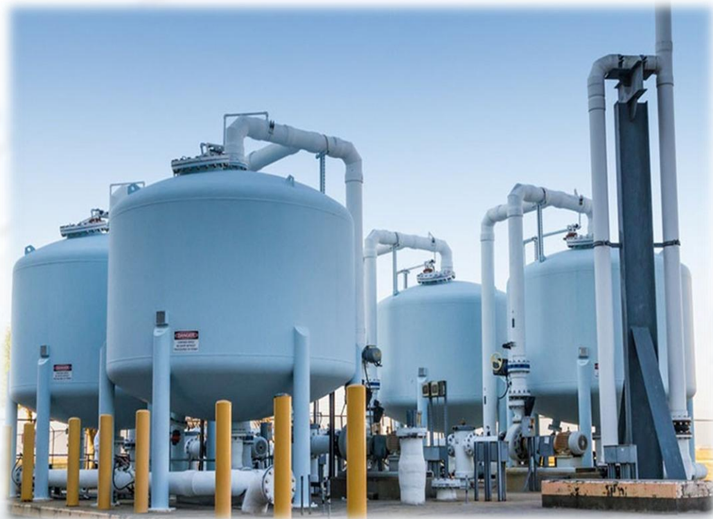
Municipal applications for Process water and Drinking Water
